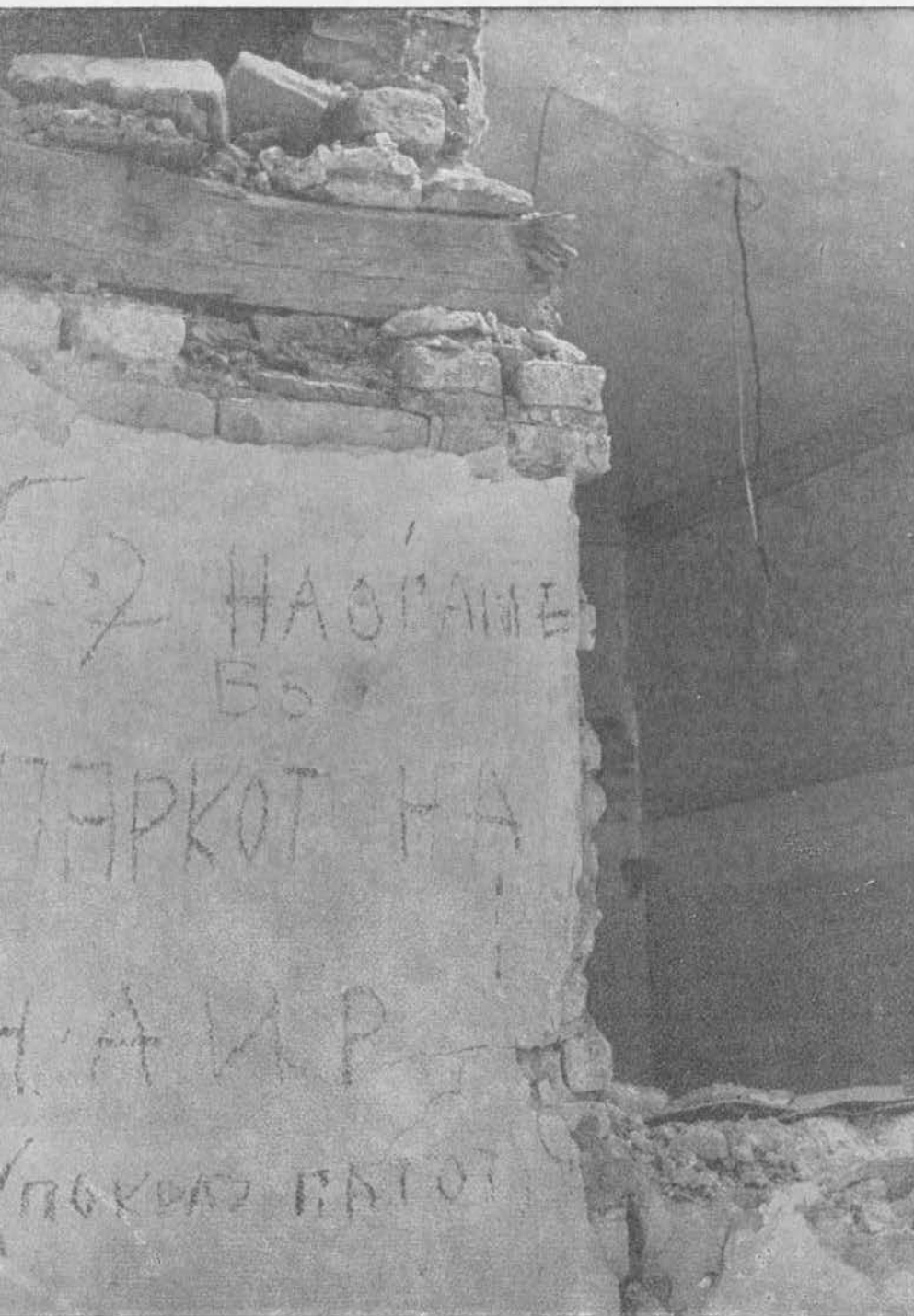
▲ THE INHABITANT OF THIS HOUSE HAD TO ABANDON HIS HOME AND LEAVE A WRITTEN MESSAGE ON THE WALL TO ALL FRIENDS AND RELATIVES CONCERNING HIS WHEREABOUTS — AT THE MOMENT IN A PARK NEAR THE SUBURB OF CAIR.
