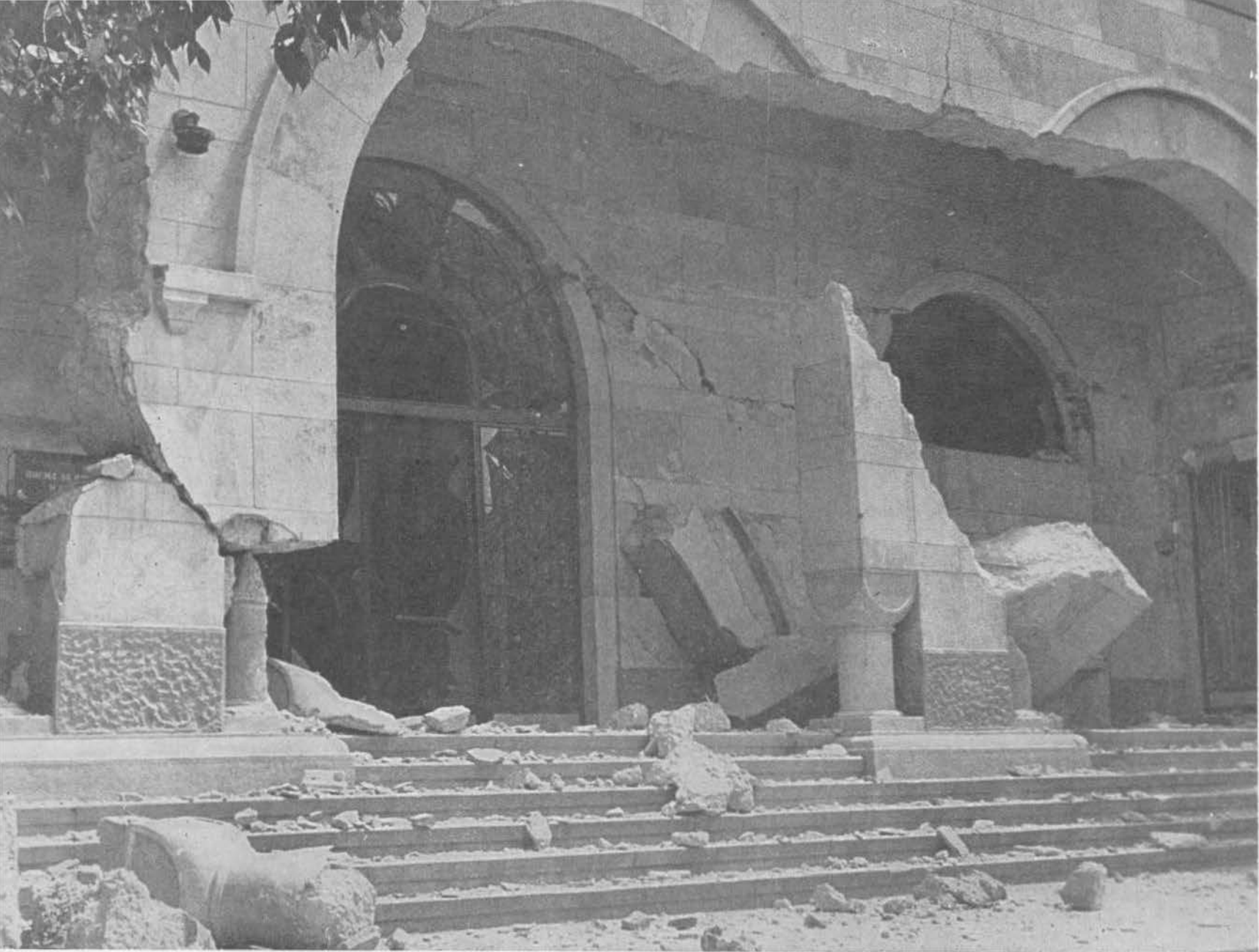
▲ THIS ENTRANCE OF POST OFFICE NO. 3 TESTIFIES TO THE BUILDING'S SOLIDITY, BUT OF THE DESTRUCTIVE POWER OF THE EARTHQUAKE TOO. IT WILL BE DIFFICULT TO REPAIR THIS BUILDING.
